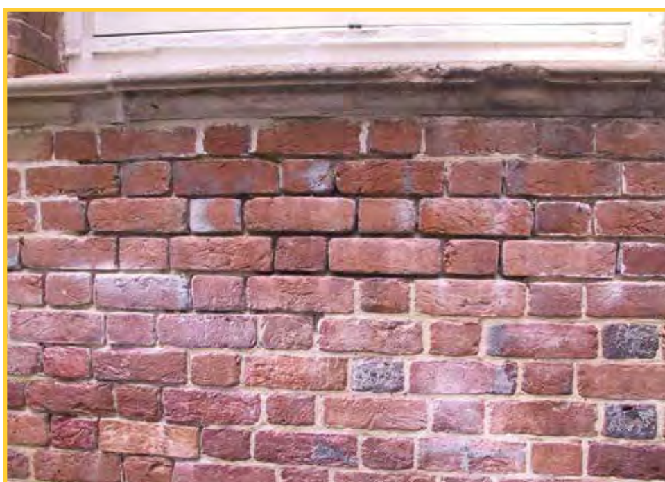
MORTAR DECAY AND SILL UPHEAVAL Salts carried upwards by rising damp cause deterioration in mortar joints and stone elements, visible here below a window on Christ Church’s southwest walls. Notice too how water has bowed both the stone sill and wooden frame.
