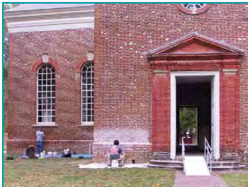
SOUTHWEST REPOINTING Rising damp tends to affect buildings more on the southern exposure, where the sun both evaporates water and pulls it higher in brick walls. Christ Church has repointed failed mortar joints along its southern walls twice in the past nineteen years (2000 and 2007, seen here). Periodic repointing may repair damage from rising damp but does not address the problem long term.
